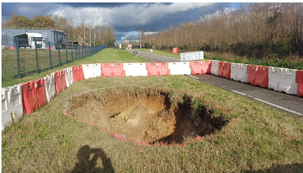
[ illustration 3 Vue effondrement 1.2 ]
